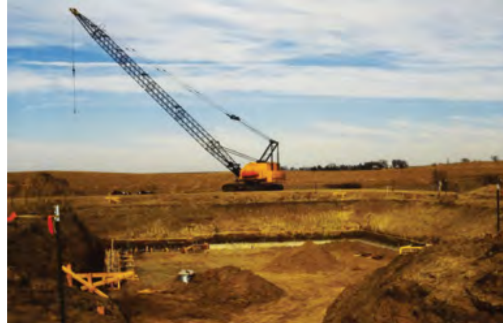
⚡ Construction begins on the lower level of the museum. Photo: Museum of Danish America.
